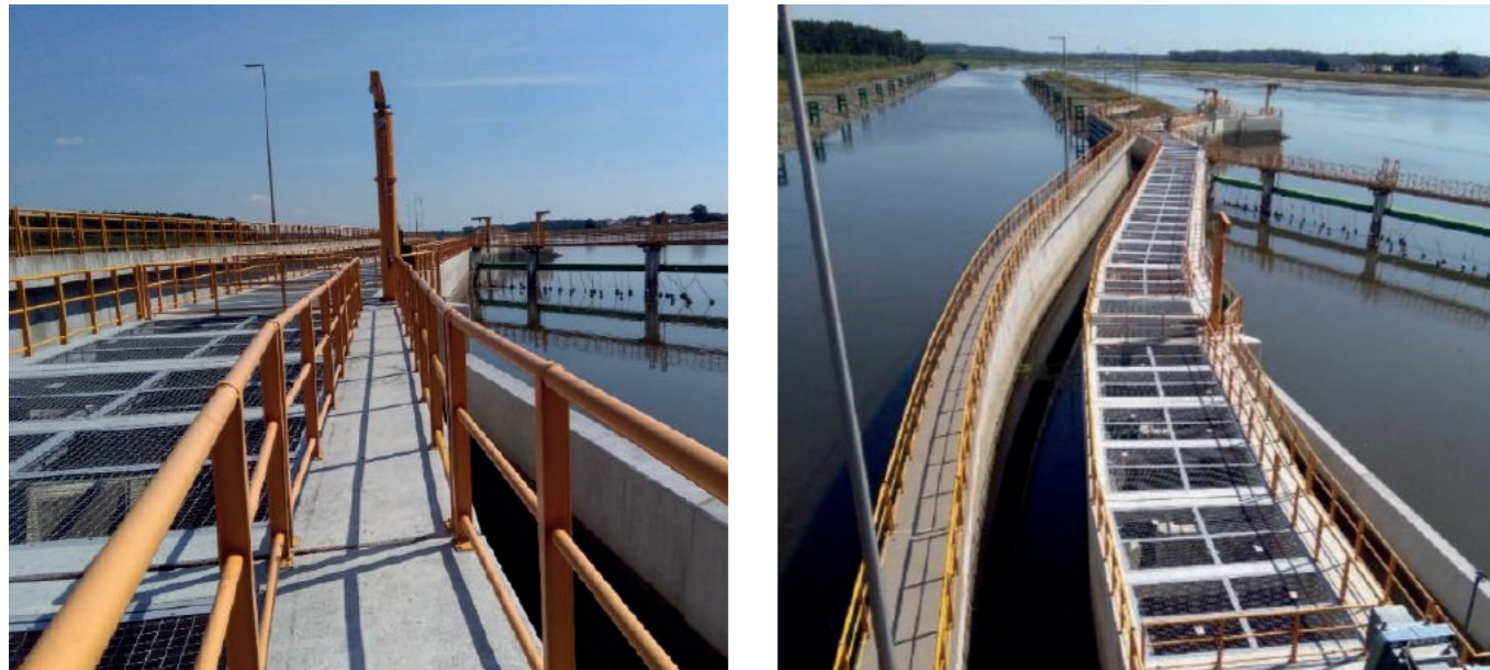
Figure 12: Fish ladder at the Malczyce barrage presented as a good example. However, this is not an action taken to achieve good water status. It is a measure to mitigate the negative impact of new hydro-technical investment – the obligation to implement it results from article 4.7 of the Directive (“all practical steps have been taken to limit the adverse effects on the status of the water body”), not from article 11. No other mitigating measures in the environmental decision enabling the implementation of this construction have been implemented. Source: International Odra draft RBMP, page 100.
